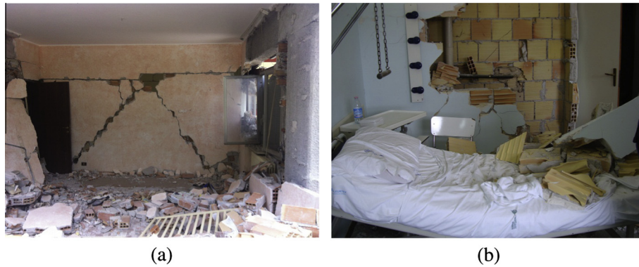
Fig. 1. Damage recorded in hollow brick partitions after 2009 L'Aquila earthquake in (a) a residential building and (b) in San Salvatore hospital.
