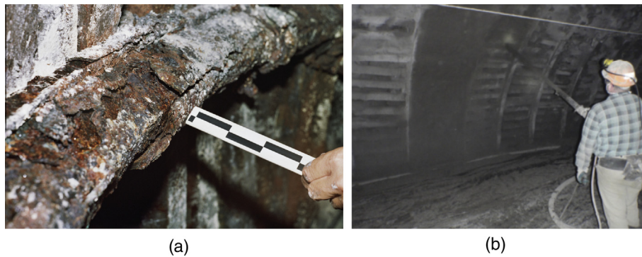
Fig. 1. Use of shotcrete in polish collieries: (a) a corroded V profile, (b) spraying a layer of shotcrete on support arches [25].
