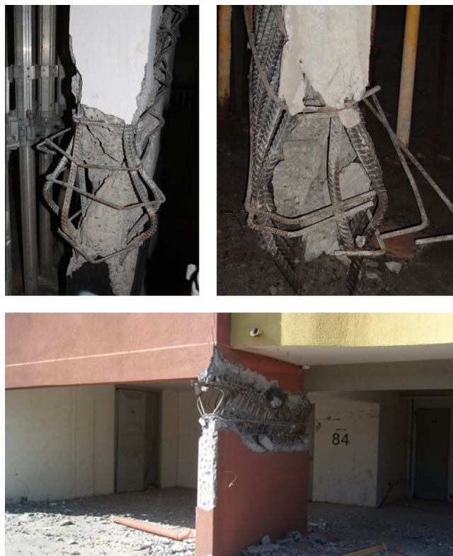
Fig. 1. Typical flexural-compressive failure of RC walls during 2010 Chile Earthquake involving crushing of concrete, vertical reinforcement buckling, and horizontal reinforcement opening.
