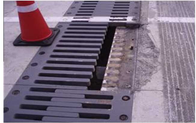
Fig. 2. Failure of the finger-joint in Young-Bong bridge II, Korea in which the right plate popped up because of the failure of the anchor bolts.
