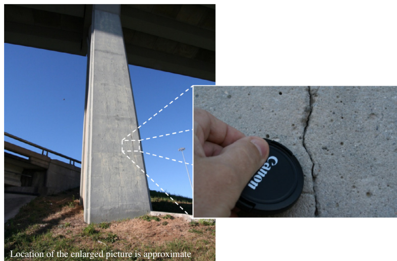
Fig. 1. Cracking in example columns due to ASR [13].
