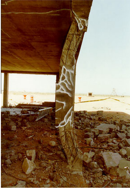
Fig. 1. RC column following a blast test [3].
