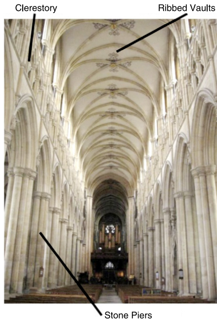
Fig. 1. The interior view of the nave of the Beverley Minster displays the limestone piers that support the stone vaulting. The leaning of the columns outwards is visually observable on site.
