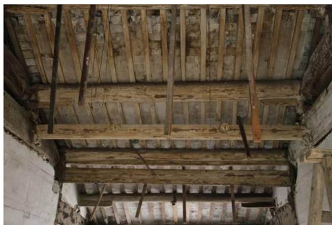
Fig. 2 Surface covered with lime.
