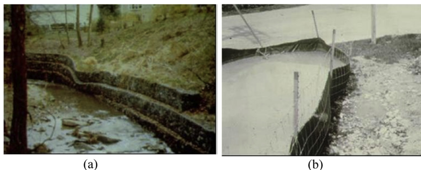
Fig. 2. Improper and proper use of woven silt film fabrics (GSI photos). (a) Gabion wall failure, (b) Silt fence success.
