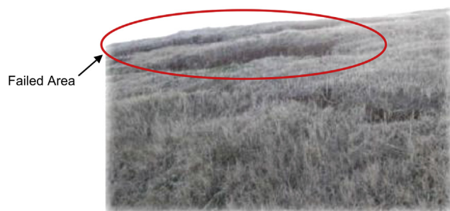
Fig. 1. Failed slope of a highway embankment in Chickasha, OK. Note: the height and inclination angle of the slope are \approx 12 m and 17^\circ , respectively.
