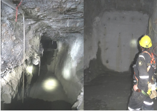
Fig. 1. A stope being backfilled (left) with a barricade constructed near the drawpoint (right).
