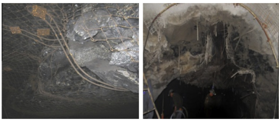
Fig. 1. Deformation and failure of the roof in the 12,501 haulage roadway.
