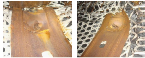
(a) Deformation and failure of shoulder coal.
