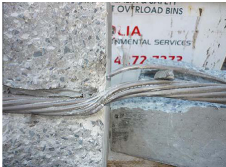
Fig. 2. Strand failure due to a combination of bending and tension and not solely due to shear [2].
