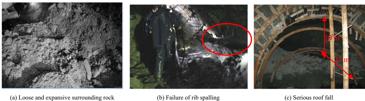
Fig. 1. Deformation and failure of the roadway.
