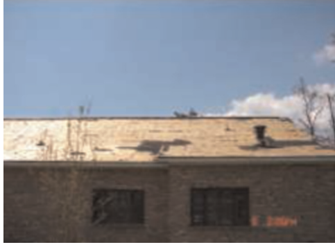
Fig. 1. Shingle loss during Hurricane Katrina, Photo#2.05-1, Courtesy: RICOWI (2007), Photographer: Bas Baskaran and John Goveia.
