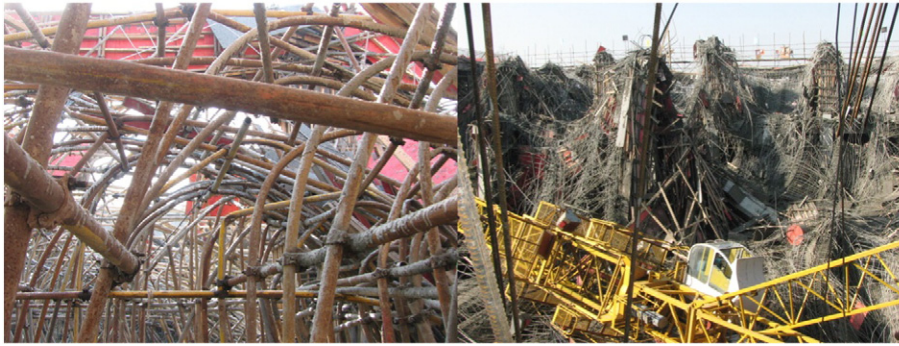
Fig. 1. Collapse of a steel tube-coupler scaffold during construction.
