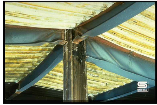
Fig. 1. Flange buckling and beam-web shear buckling in combination [7].
