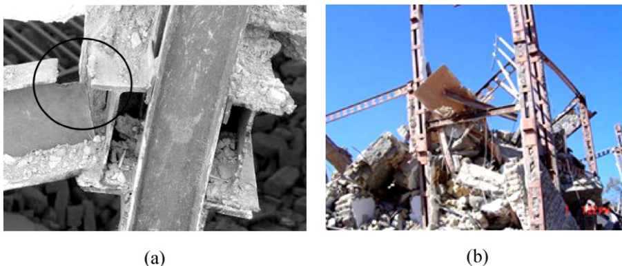
Fig. 2. Brittle saddle connections failure — total collapse examples in Bam earthquake (Mw. 6.5, 2003) [1].
