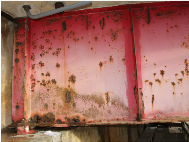
(a) Pitting corrosion
