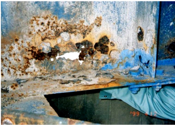
(b) Through-thickness pitting corrosion [6]
