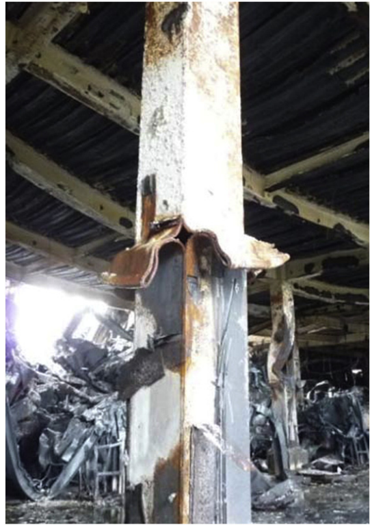
Fig. 2. Failure of PJP box column in the fire event. (Courtesy of C.P. Chen).
