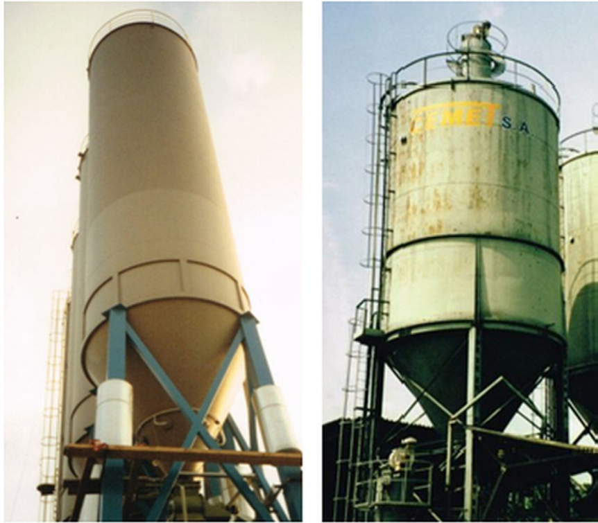
Fig. 1. Examples of stiffened, column supported steel silos with the use of transition ring over short ribs.
