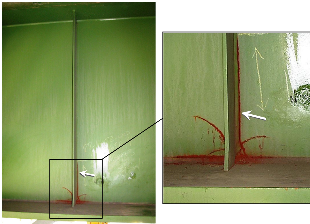
Fig. 1. Crack along fillet weld at gap between I-girder web and welded stiffening plate.
