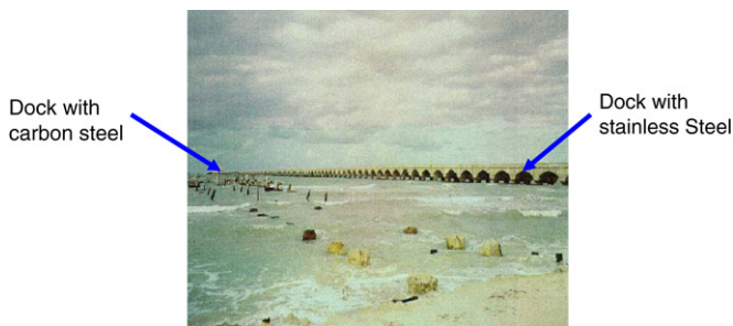
Fig. 2. View of the dock constructed with stainless steel (right) and carbon steel (left) [4].
