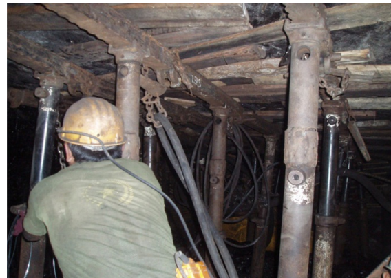
Fig. 4. Steel longwall supports with friction props and articulated caps.
