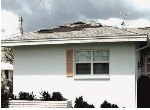
Fig. 1. Example of asphalt shingle roofing damage (Punta Gorda, FL, Hurricane Charley, 2004)
