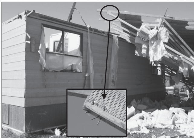
Fig. 1. Photograph of a global roof failure in Saskatchewan, Canada, on July, 4, 2010.
