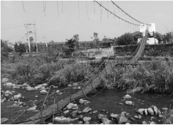
Fig. 1. Snapping of steel suspender wire ropes.
