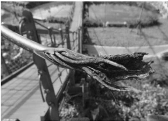
Fig. 2. Snapped steel wire covered with plastic materials.
