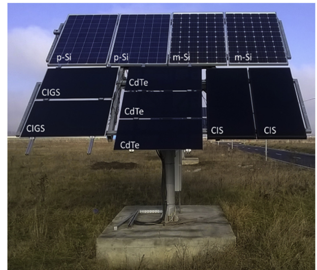
Fig. 1. Platform P2 with five types of PV modules.
