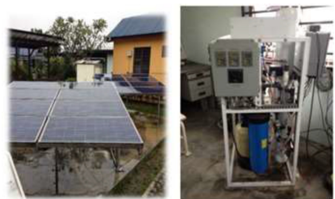
Fig. 1. Photo of PV and RO test units located in the solar field @UKM, Malaysia.
