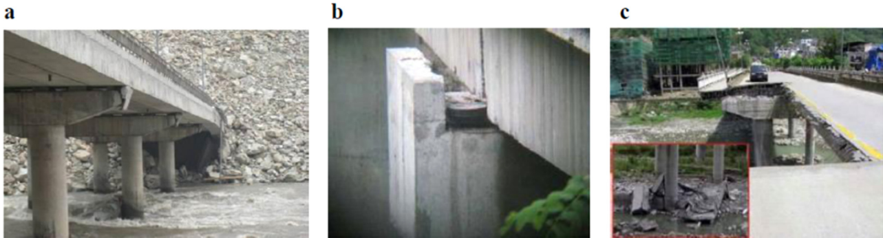
Fig. 2. Typical damages of highway bridges during Wenchuan earthquake: (a) shear key failure, (b) bearing sliding, and (c) span collapse.
