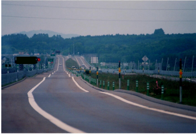
Fig. 1. Typical differential settlement of road embankment constructed on peaty ground.
