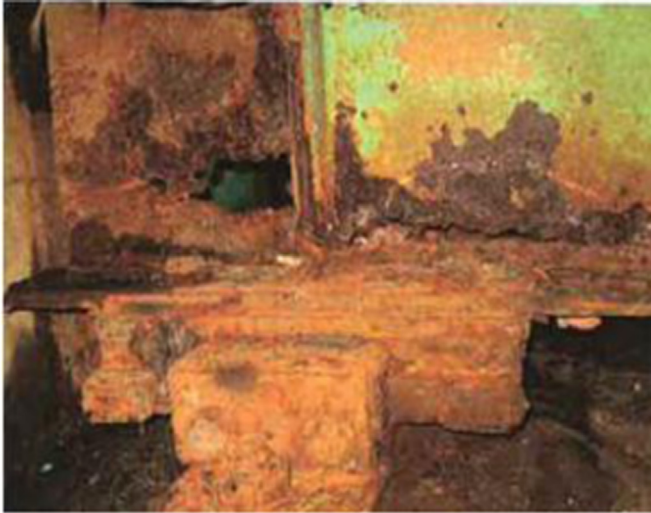
Fig. 1. An example of local corrosions in end panels [15].
