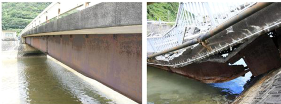
Fig. 2. Collapsed plate girder bridge reported by Ahn et al. [6].
