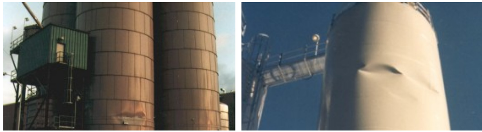
Fig. 1. Two instances of local dent-shaped irregularities on steel shell structures [18].
