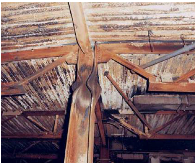
Fig. 1. Local buckling in a typical steel columns.
