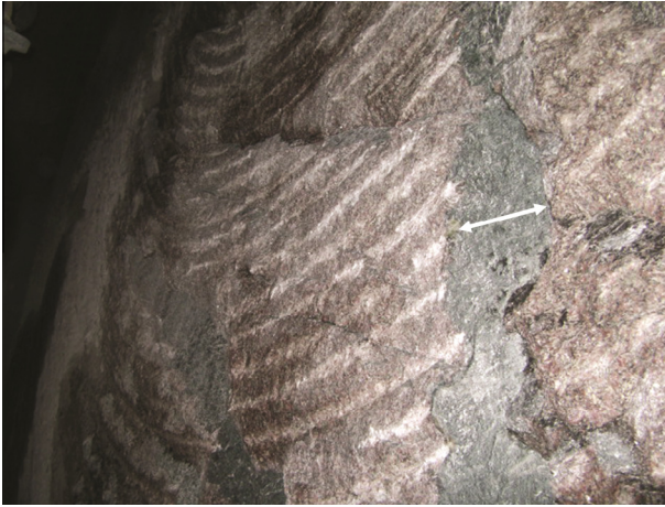
Fig. 1. TBM heading face with blocky rock mass which appears to have moved on discontinuities (arrow) after boring. Image courtesy of The Robbins Company (Home, 2009).
