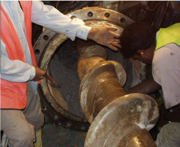
Fig. 1. Abraded screw conveyor from an EPB TBM.
