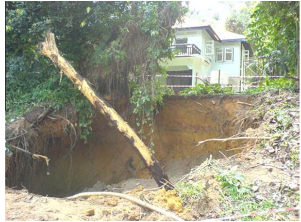
Fig. 4. Sinkhole over a slurry TBM drive.
