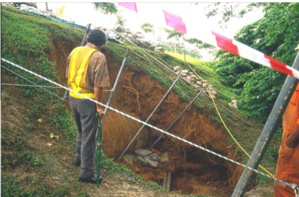
Fig. 3. Sinkhole over an EPB TBM drive.
