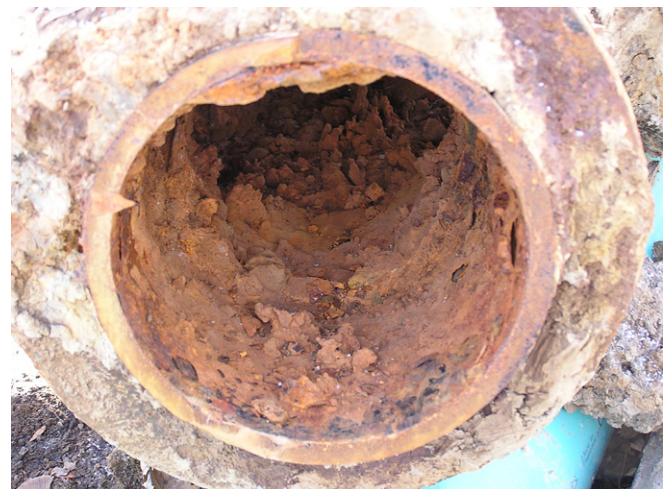
Fig. 1. A typical corroded water main from the City of Hamilton.
