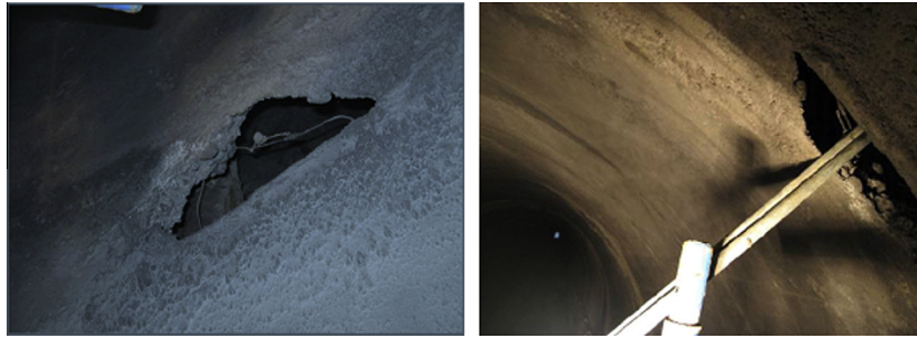
Fig. 1. Photographs of voids behind the tunnel lining (Liu, 2007).
