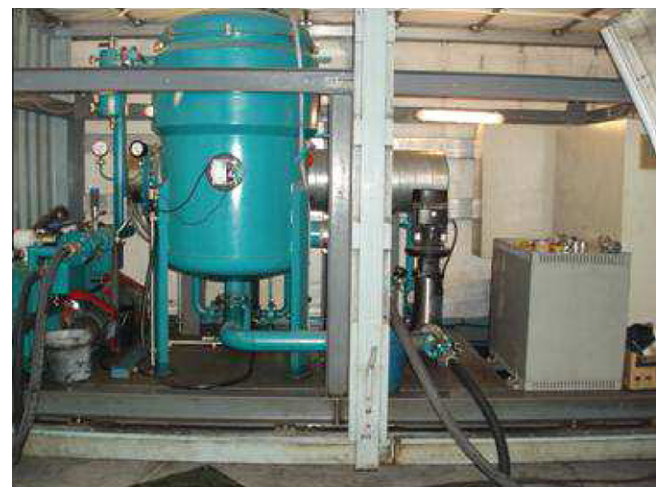
Fig. 3. Oil treatment equipment.
