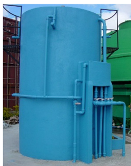
(b) UASB reactor
