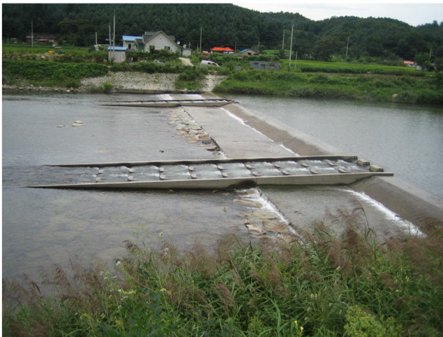
(b) Fishways installed at Dangmugae weir in Gapyeng stream
