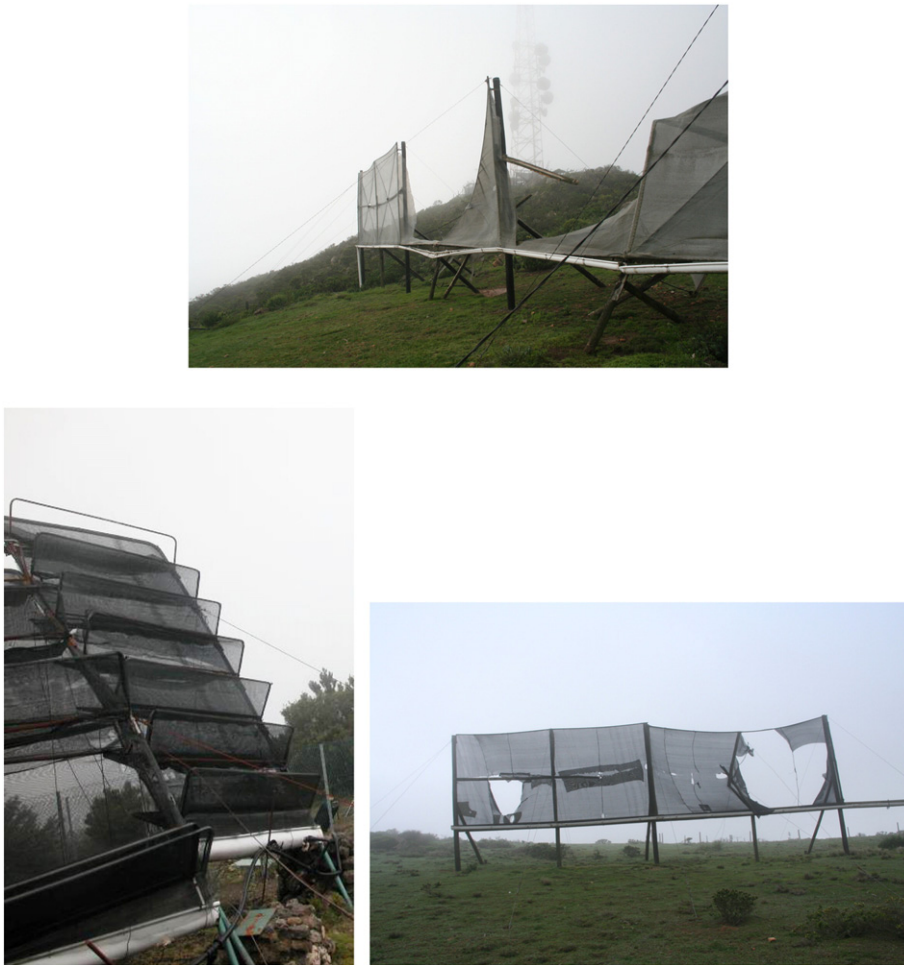
Fig. 1. Failure of large fog collectors: (top; Peña Blanca, Chile) failure of the supporting structure; (bottom, left; Anagua project – Canary Island, with permit by Carlos Sanchez Recio) failure of the foundation; (bottom, right; Peña Blanca, Chile) breakage of the mesh.
