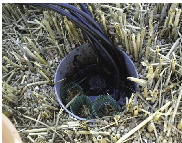
Fig. 1. Microbial fuel cells implemented within the wetland at the beginning of the experiment.
