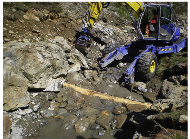
Fig. 2. Photo showing the works by the Dept. of Hydraulic Engineering of the Autonomous Province of Bolzano for the installation of the acoustic pipe in the Saldur River (section LSG, May 2011). Stream water was diverted to place a wooden log on the channel bottom, later stabilized by large rocks forming a ramp. The acoustic pipe was then fixed to the log by metal braces. A semi-circular slot – visible in the image – had been previously carved to host approximately half the diameter of the pipe.
