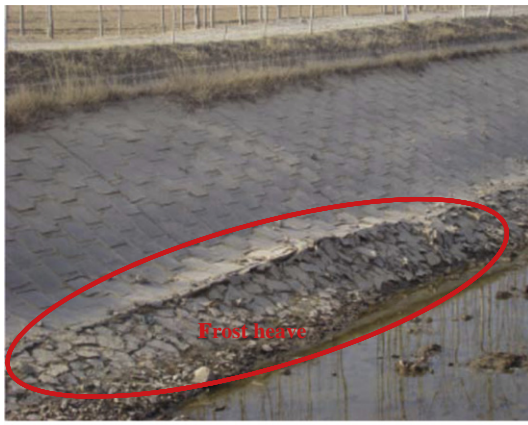
(a) Frost heave damage
