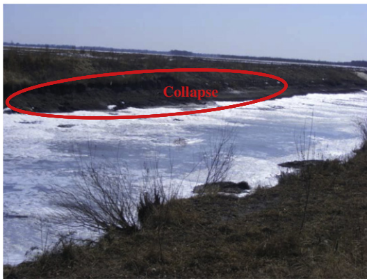
(b) Collapse of canal slope
