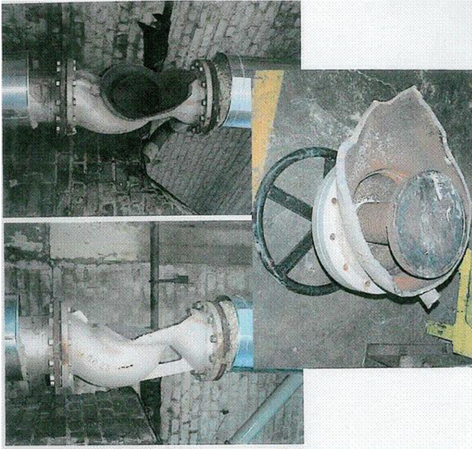
Fig. 1. Examples of pipeline damage caused by water hammer.
