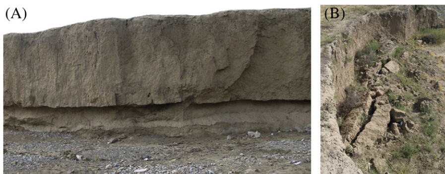
Fig. 1. (A) Fluvial erosion at the toe of a riverbank (bottom layer) results in the formation of an overhanging profile in cohesive banks of the Kordan River. (B) Destruction of the overhang from cantilever failure.
