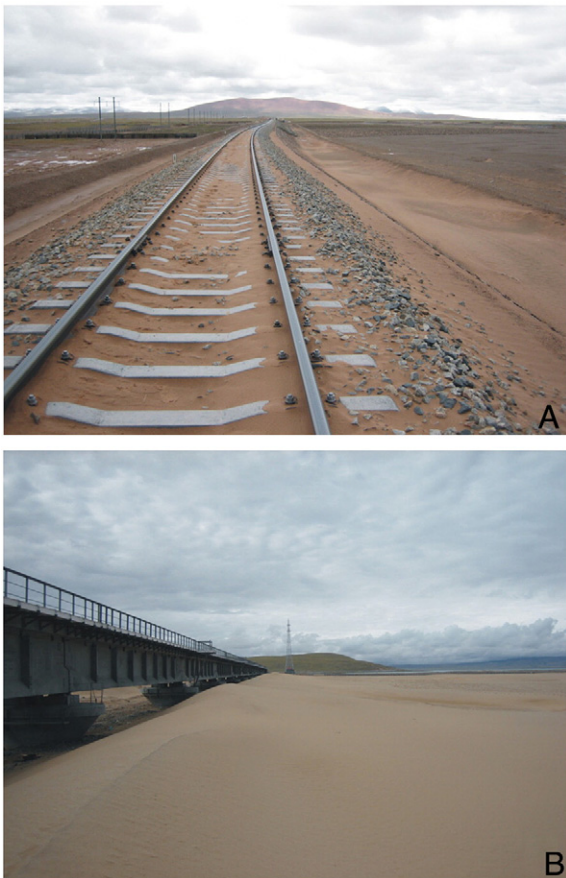
Fig. 2. Typical damage caused by windblown sand along the QTR at (A) Xiushuihe, and (B) Cuonahu.
