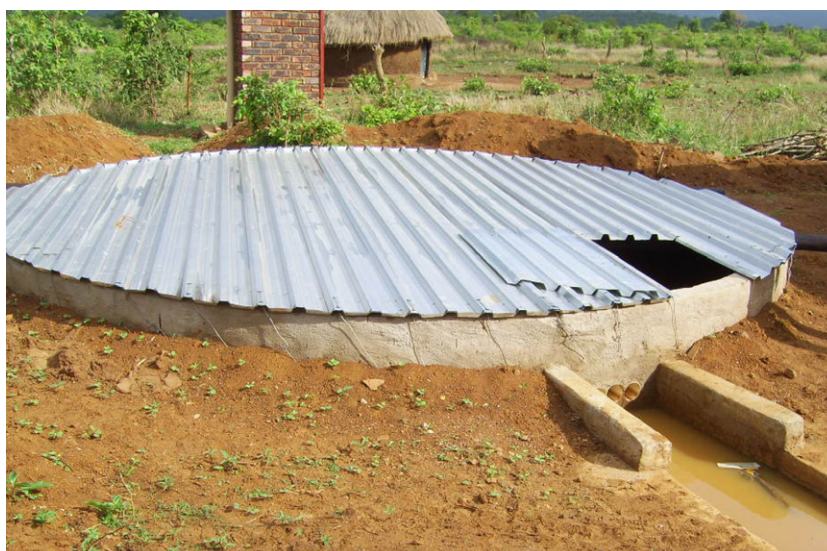
Fig. 1. 30 m 3 RWH underground tank constructed by under the DWAF demonstration phase (Picture by Papenfus).
